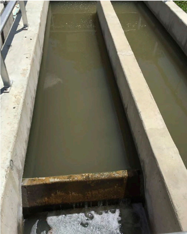
Appendix 5: Chlorination Chamber
